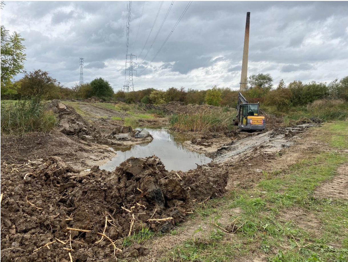
Figure A2-14: Dredging management in ponds illustrating how management strategy can be improved for biodiversity
